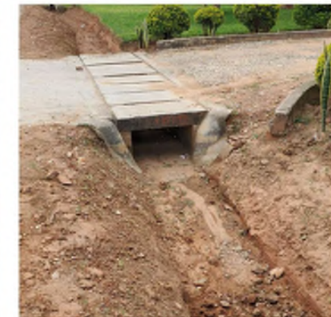
PI-d: Small Box Culvert concrete box culvert for crossing small wadi/ravines, note removable blocks for cleaning
