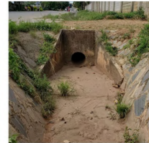
PI-b: Small Pipe Culvert concrete pipe culvert with stone reinforced channel for small wadi/ravines
