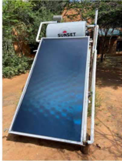
PI-f: Example Solar Hot Water Heater Solar Geyser at CCF Namibia.
