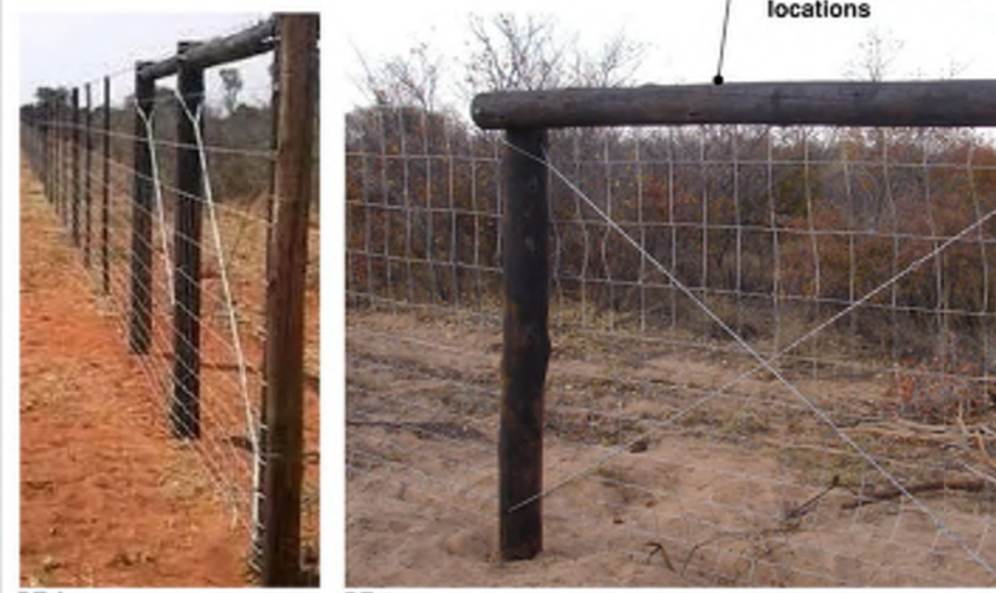
PF-f PF-g 1000mm Bonnox Fence Precedent: use cap rail at viewing/leaning locations and at ends for bracing
