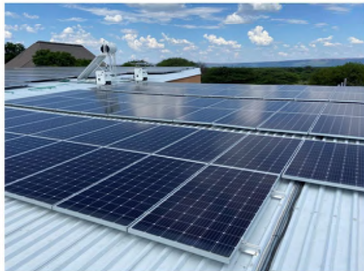
PI-h: Example Solar Panel Array CCF Namibia rooftop solar array. A large area(s) will be required for keeping the solar panels required for power production.
