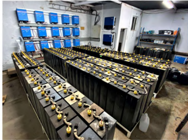
PI-g: Example Battery Room CCF Namibia battery room. Multiple battery banks and inverters supply electric to the center campus. Main switch board for campus is located in the rear of the room.
